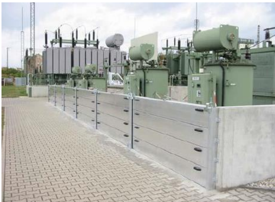
Figure 6.5: removable flood panels (ENA ETR138 Annex 1)
