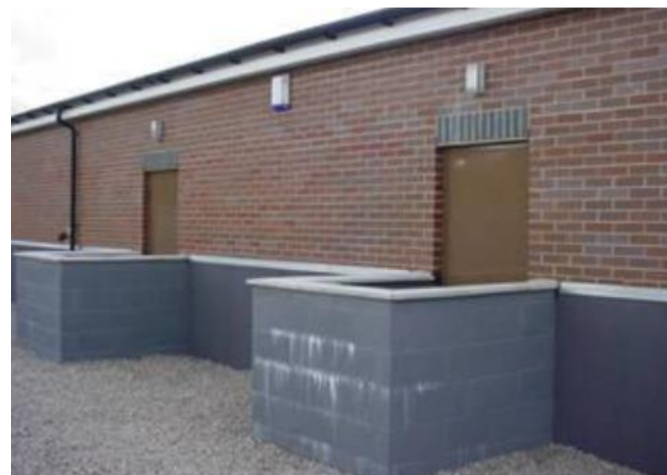
Figure 6.4: Exterior of building displaying flood protection and bunding to access and emergency exit doors (ENA ETR138 Annex 1)
