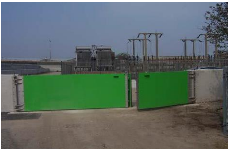
Figure 6.6: Flood protection gates (ENA ETR138 Annex 1)
