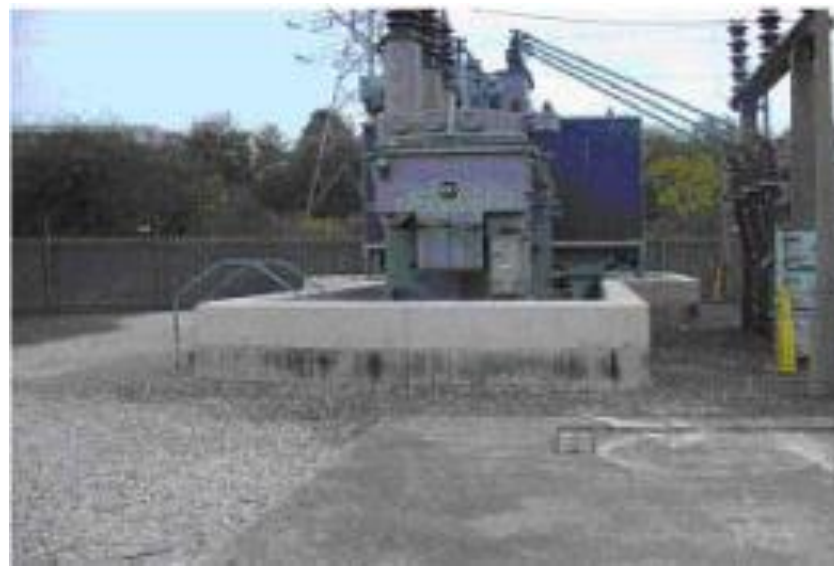
Figure 6.1: Raised bund and access platform around a transformer
